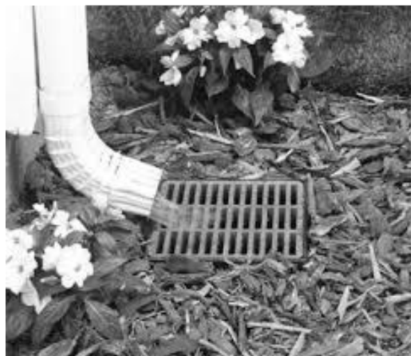
Inlet Box with a Grate
